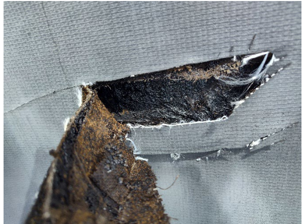
Photo 8: View of the asbestos containing black/brown flashing on the roof parapet walls.
