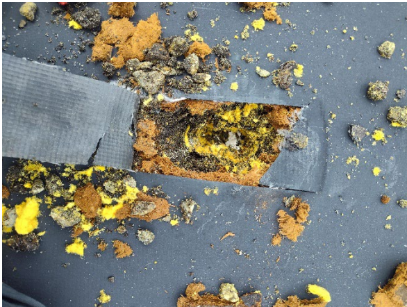
Photo 9: View of the black roofing, brown insulation, yellow insulation, and asbestos containing black/brown flashing on the roof.
