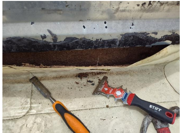
Photo 10: View of the asbestos containing black tar on the base of the HVAC unit and roof hatch.
