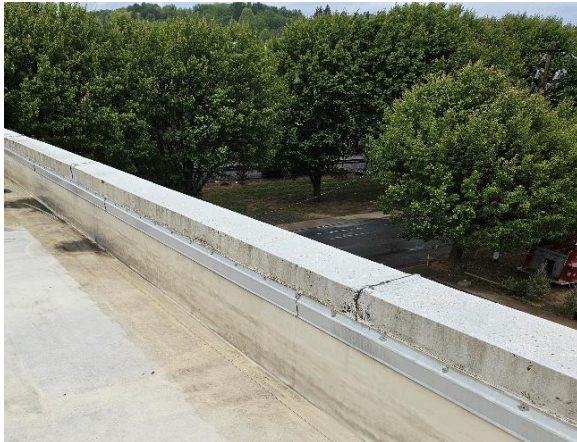
Photo 7: View of asbestos containing white/black tar on the roof parapet wall seams.
