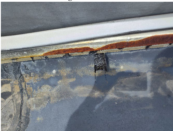
Photo 11: View of the asbestos containing black flashing on the base of the roof HVAC units and roof hatch.
