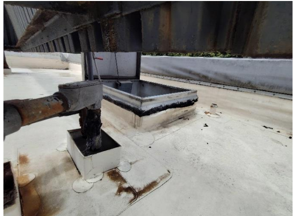
Photo 8: View of the asbestos containing black tar on the metal wall base on the roof.
