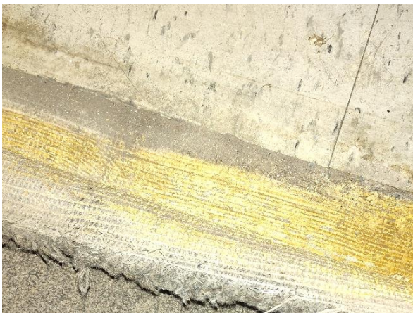
Photo 5: View of the asbestos containing off-white floor tile and underlying black mastic in the second-floor hallway and office area.
