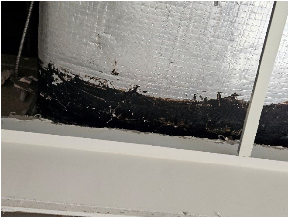
Photo 7: View of the asbestos containing black mastic on the HVAC ductwork in the ceiling.
