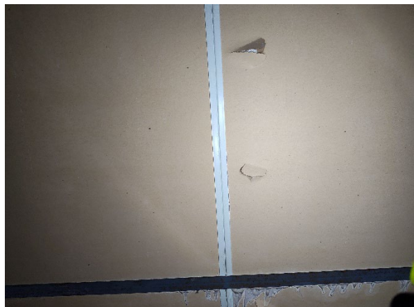
Photo 6: View of the absence of joint compound on the drywall.
