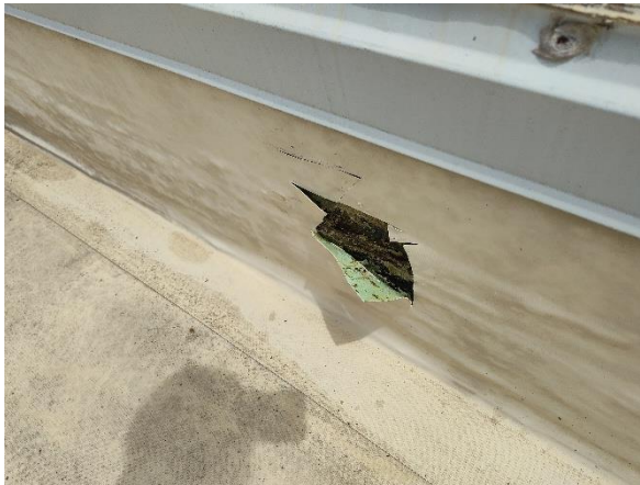
Photo 9: View of the asbestos containing black tar paper on the roof parapet walls.
