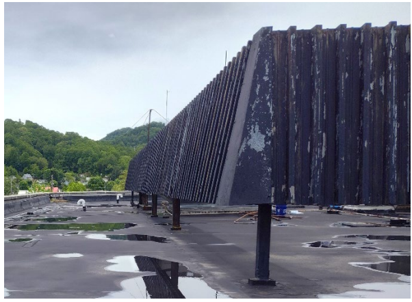
Photo 10: View of the asbestos containing black tar on the base of the metal wall on the roof.
