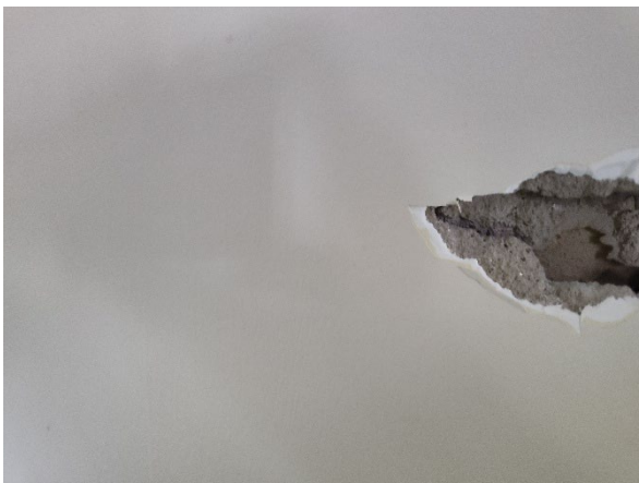
Photo 5: View of the white plaster skim coat and gray plaster base coat on the walls throughout. Note the drywall behind.
