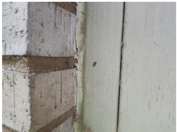
Photo 6: View of the asbestos containing beige caulk on the exterior door frames.
