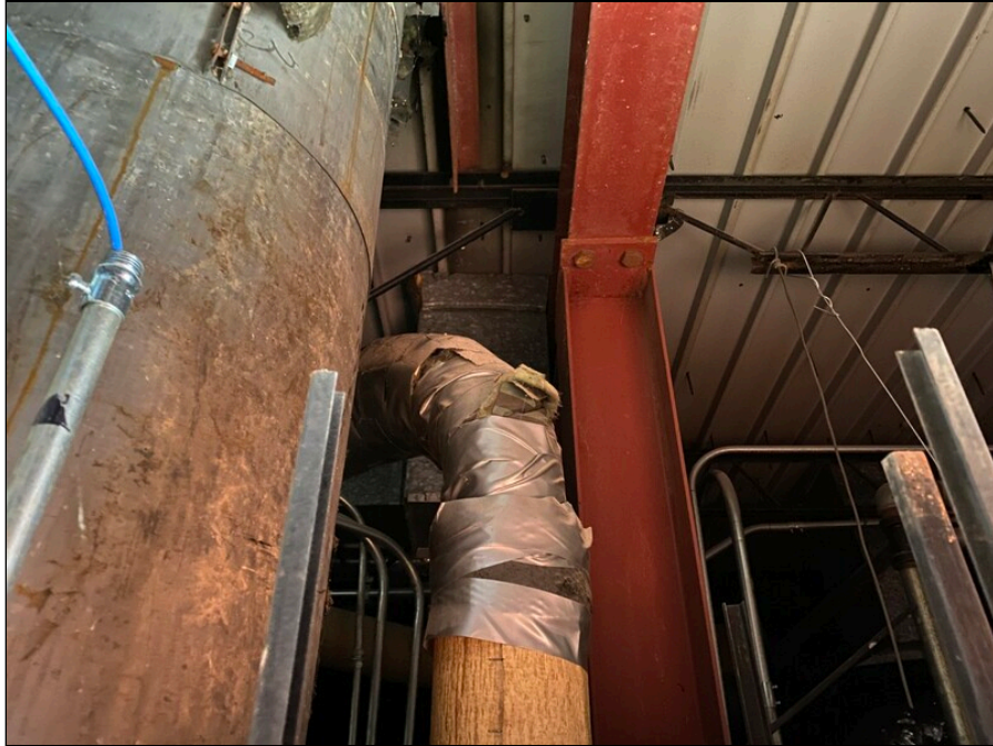
7 - View of fiberglass piping.
