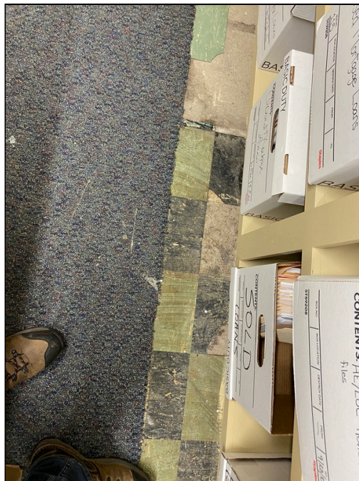
4 - View of asbestos-containing black floor tile
